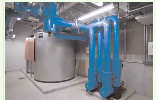
Ice Storage System
