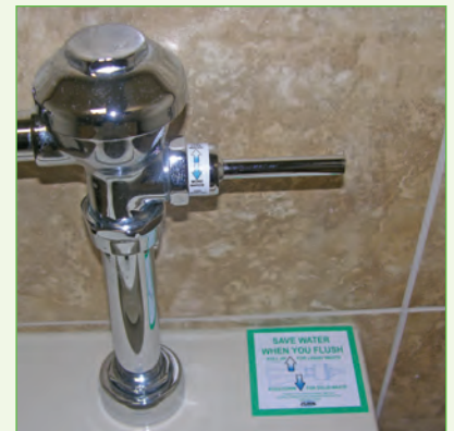
Efficient Bathroom Fixtures
