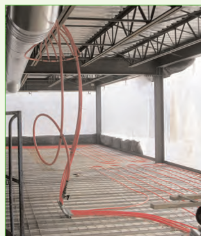
In-Floor Radiant Heating
