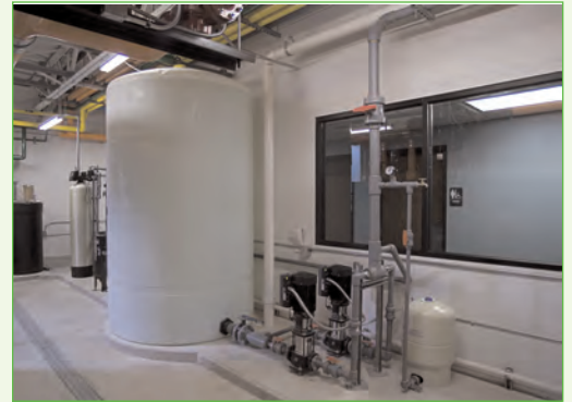
Greenwater Reclamation System
