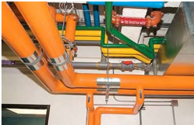
Colored pipe offers visual clues to office visitors touring the green expansion: blue = chilled water; orange = heated water; green = domestic cold water; and yellow = domestic hot water.
