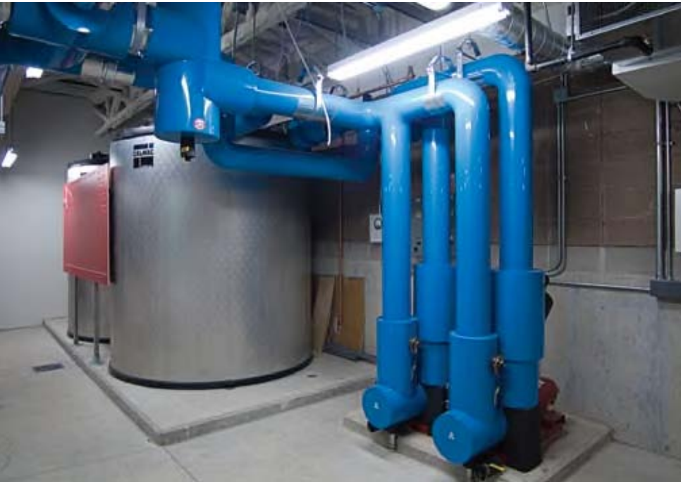
The "icemaker" works at night when electricity rates drop by half and works in tandem with a traditional chiller.
